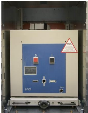
CB in Test Position
